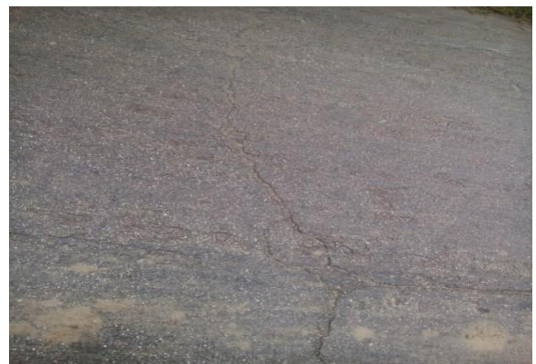
Figure 6 Transverse cracking at Dastur Nagar
