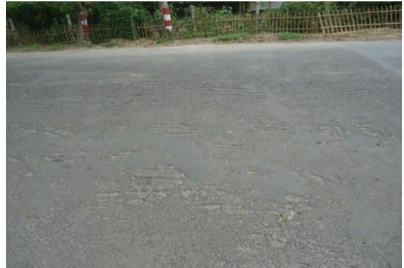
Figure 5 Slippage cracking at Chaprashhi Pura
