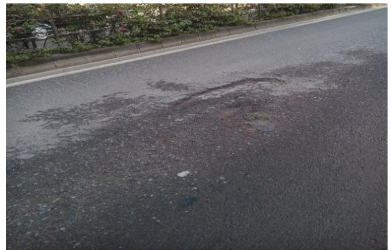
Figure 10 Water bleeding at Rayba Hotel
