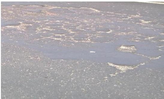
Figure 4 Block cracking at Laali Lawn
