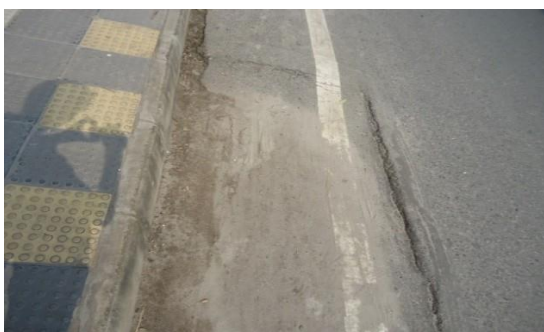
Figure 13 Rutting at Nowdapara
