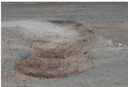
Figure 8 Potholes at Juni Vasti
