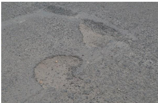
Figure 12 Depression at Yashoda Square
