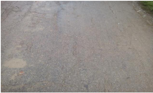
Figure 7 Longitudinal cracking at Yashoda Square
