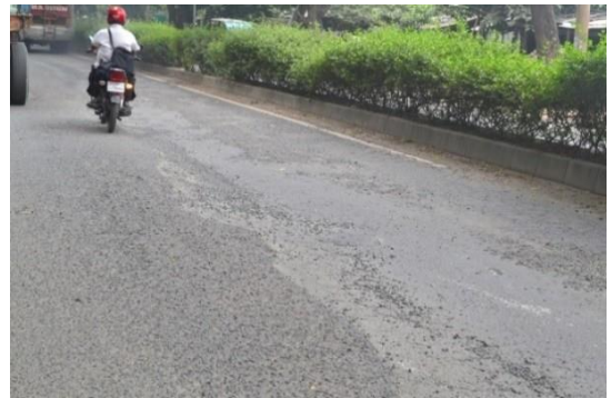
Figure 9 Raveling at Yashoda Square
