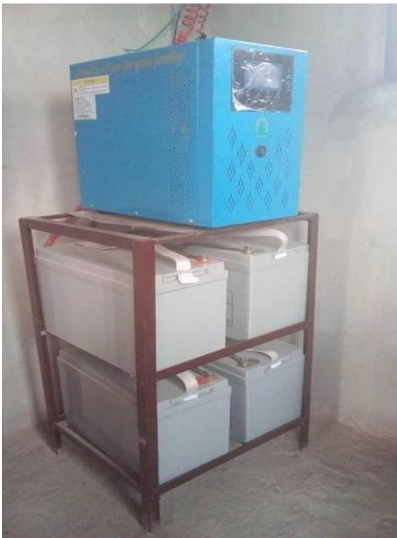
Fig 3: Array of Batteries and Inverter.
