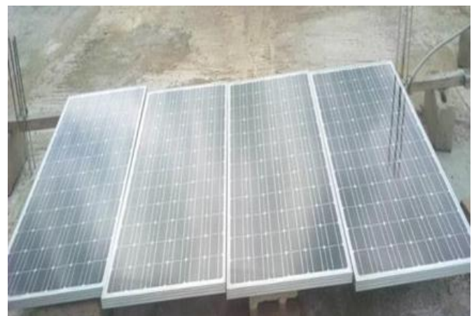
Fig 3: Array of PV panels.
