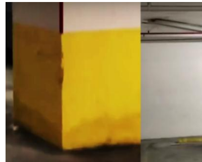
Fig -16: Enhanced image of water pulling into columns.
