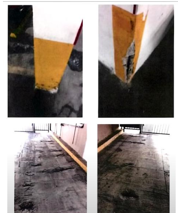
Fig -7: Spalling of concrete from garage columns and garage floor.
