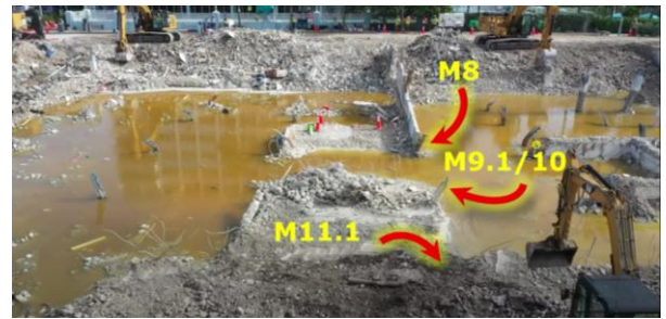
Fig -15: Waterlogged beneath the floor of the garage.
