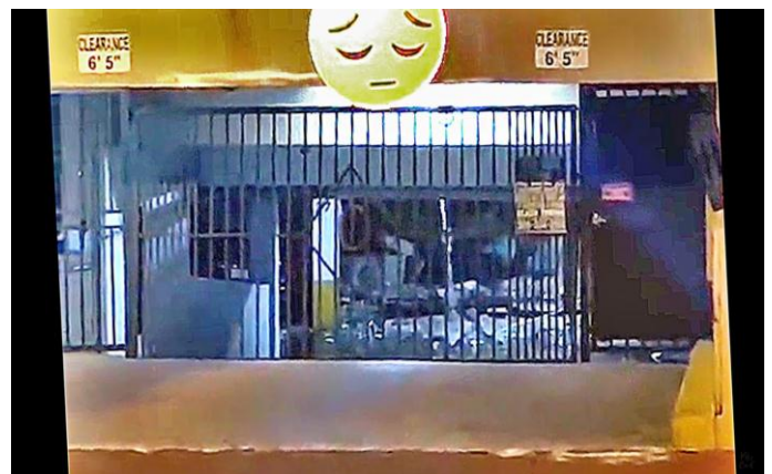
Fig -21: Big chunks of concrete on the floor of the garage.
