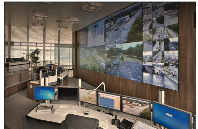
Figure 1: TMC [Traffic Management Center]
