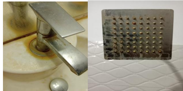
Fig -1: Effect on ceramics and steel fittings due to excess iron content and hardness in domestic water
