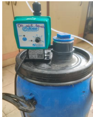
Fig - 7: Dosing Pump installed
