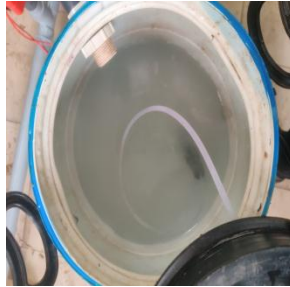
Fig - 9: Chlorine Tank
