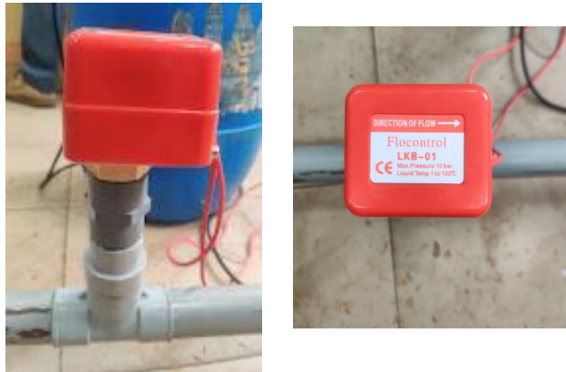
Fig - 5: Flow switch installed in the model
