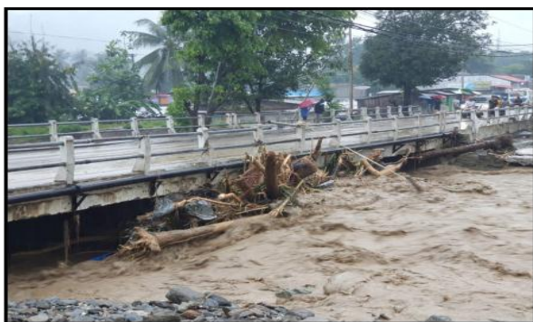
Fig -4: Debris deposited at the bridge
