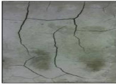
Fig -5: Kraai method crack pattern
