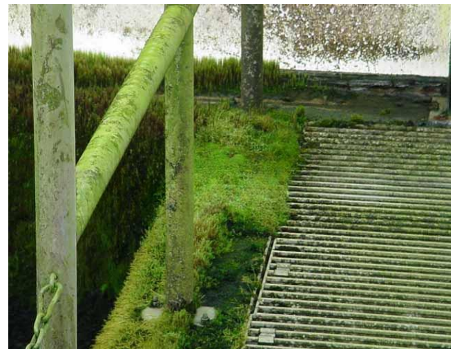
Fig -8: Algae Growth Cooling Tower
