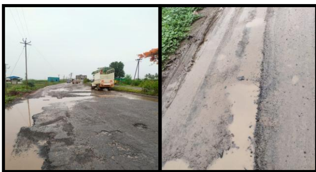
Fig 7 : No Drainage system
