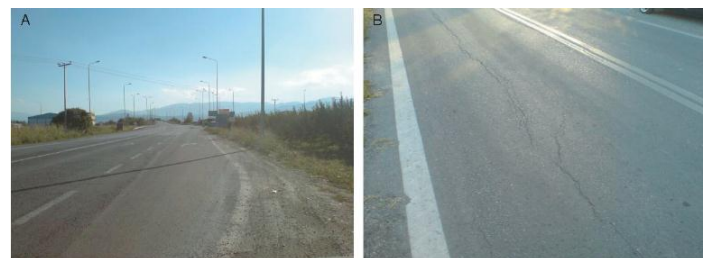
Figure 3: Inadequate super elevation and curve radius in NH 353-J
