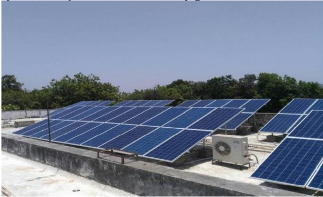
Fig -4: Solar Power Plant
