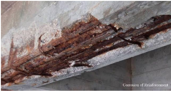
Fig-3: Crack occur due to Chemical Reaction between concrete and steel [reinforcement].
