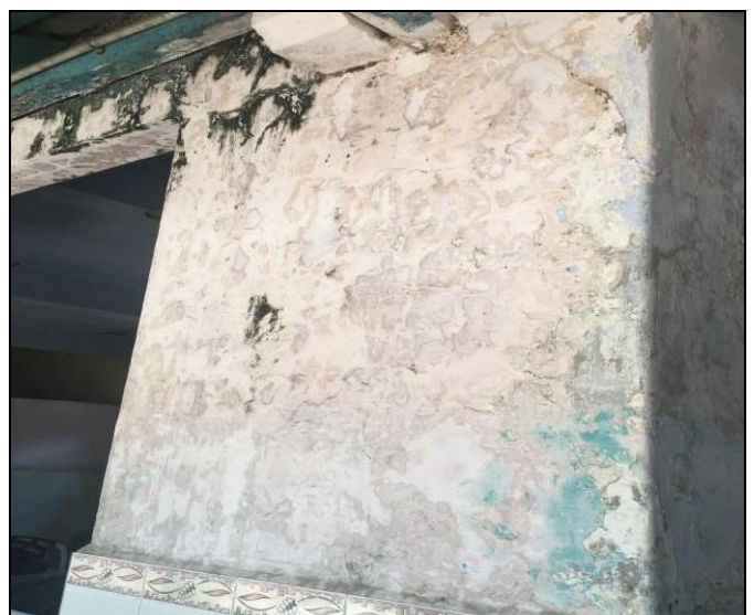
Fig -4: Dampness in columns
