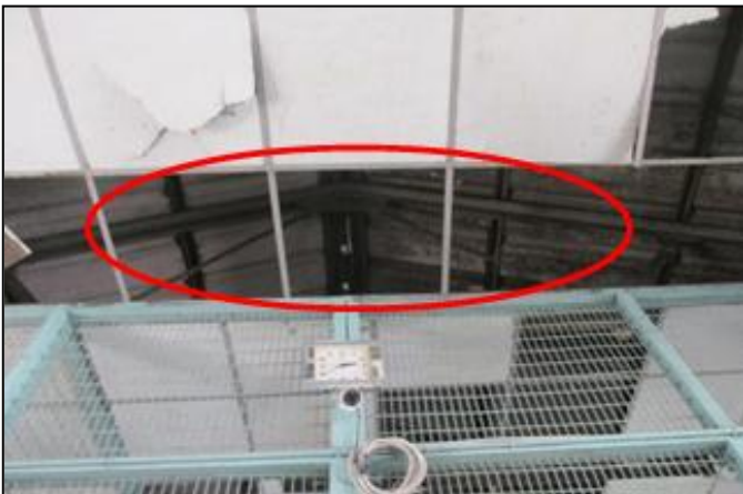
Fig -6: Damaged false roofing and Truss
