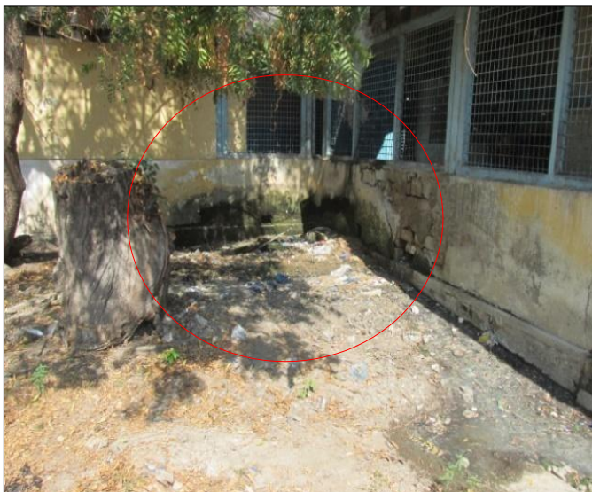
Fig -1: No Plinth Protection
