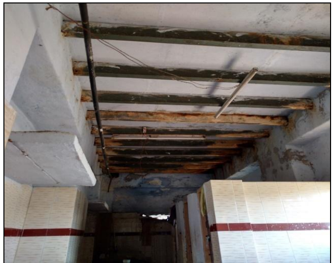
Fig -3: Distressed in wooden members
