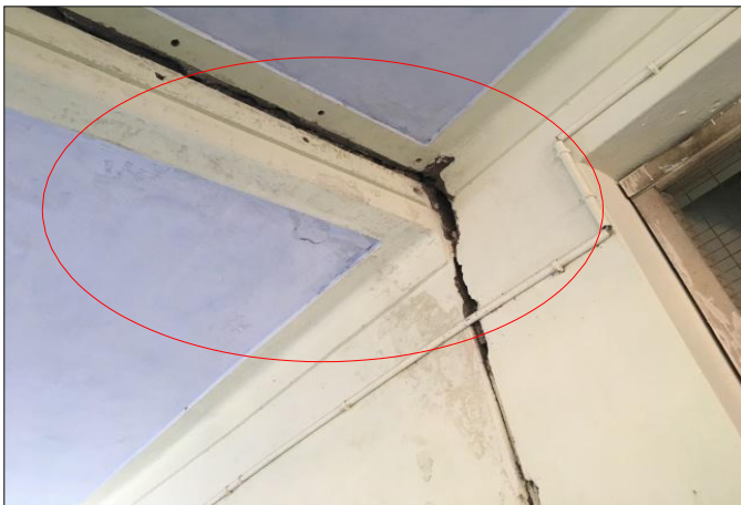
Fig -5: Cracks near Expansion Joint
