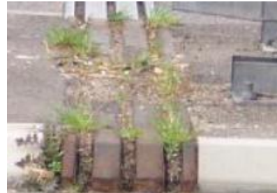
Fig -13: Vegetation growth seen in expansion joint
