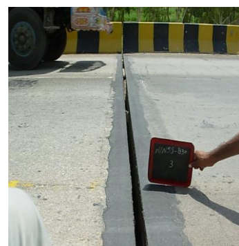
Fig -15: Debris build up in the seal in the expansion joint
