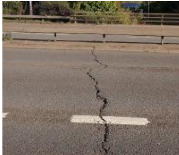
Fig -10: Improper injection of sealants
