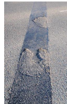
Fig -14: Loss of Asphaltic plug material
