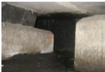
Fig -11: leakage of joint near pedestal
