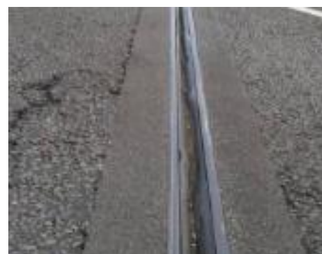
Fig -9: Rutting of wearing surface
