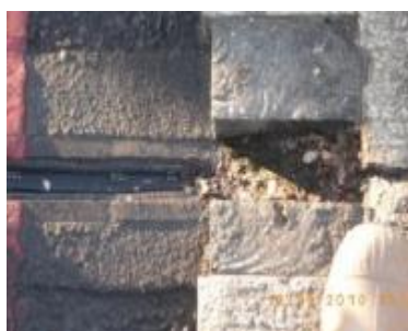
Fig -12: Damaged fixtures in expansion joint
