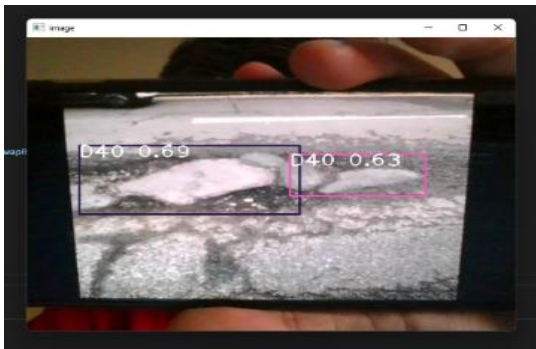
Fig -9: Pothole Accuracy of 69% and 63%
