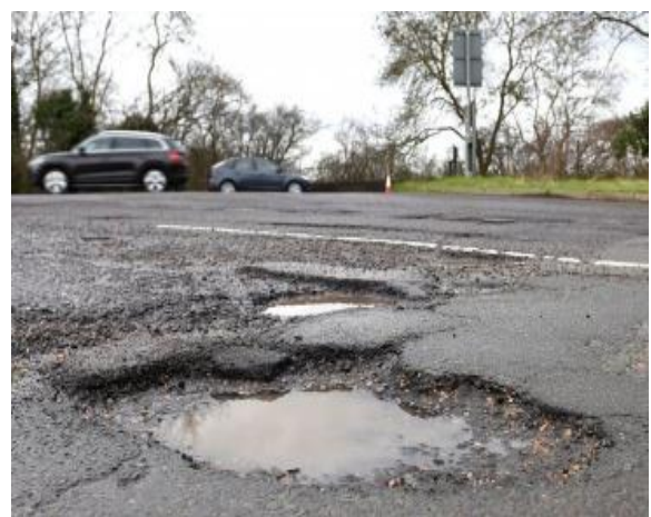
Fig -1: Conditions of roads with potholes.
