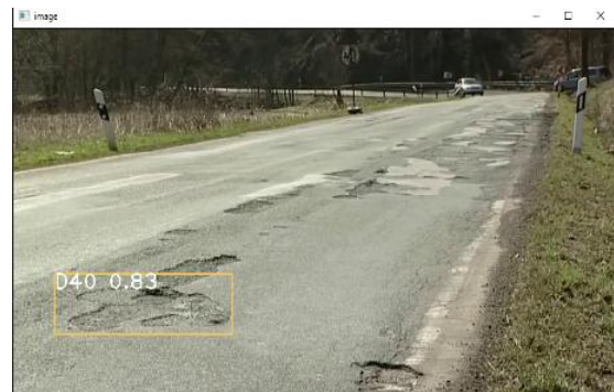
Fig -8: Result image of Detected pothole (2) Class Label: D40, Accuracy achieved: 83%
