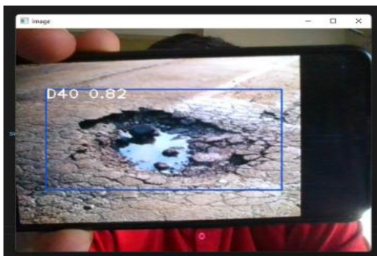
Fig -7: Result image of Detected pothole (1) Class Label: D40, Accuracy achieved: 82%
