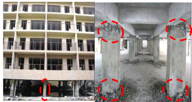
Figure 4. Plastic hinged formation at column ends of the ground storey columns in China Earthquake 2008
