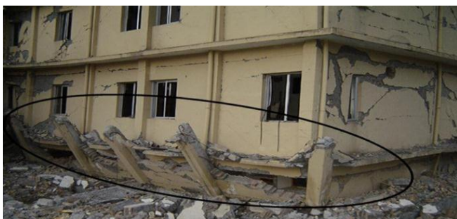
Figure 3. Shear failures of ground storey columns (Ref: World Housing Encyclopedia, EERI & AIEE)
