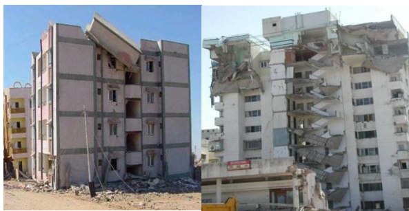
Figure 2. Failure of the OGS buildings in Bhuj Earthquake (Ref: www.nicee.org)
