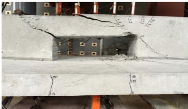
Fig -3: Crack pattern at ultimate state
