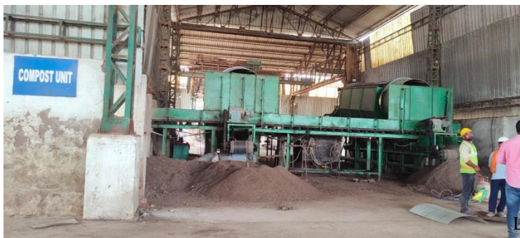
Figure5: Processing Plant, Shivari Mohan Road (source: site visit, 2022)
