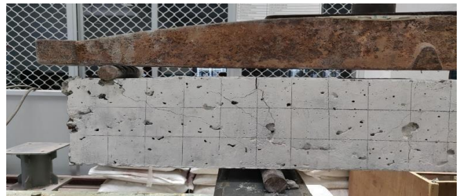
Figure -5: Crack development in Beam without curtailed reinforcement
