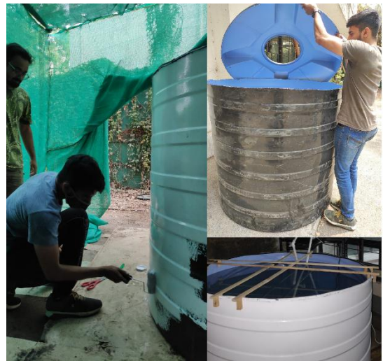
Fig 14: Modification of tank by removal of upper section and painting it white to maintain the system temperature
