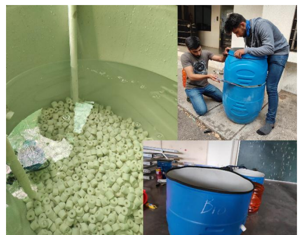
Fig 18: Removing excess part of the tank and introducing bio media for setting up the biological filter
