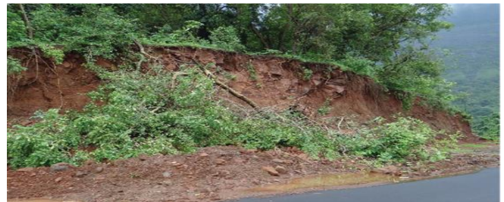
Figure 11. Case 1 Typical locations on existing road where PCC and RCC retaining walls can be proposed on valley side
