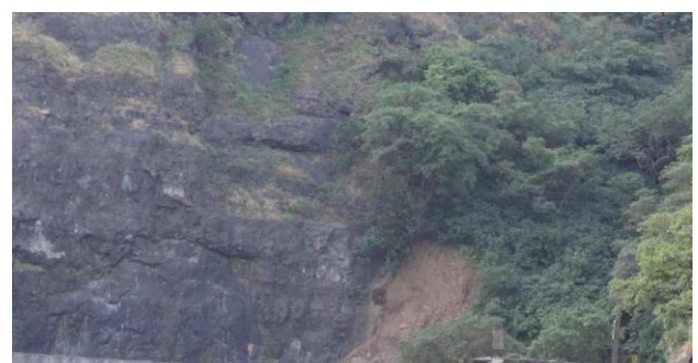
Figure 14. Case 4 The slope downhill is to be protected for further deterioration. The risk involved is of washing away the road all sudden.
