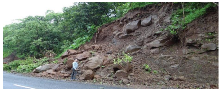
Figure 12. Case 2 Typical locations on existing road where Gabion wall can be proposed.
