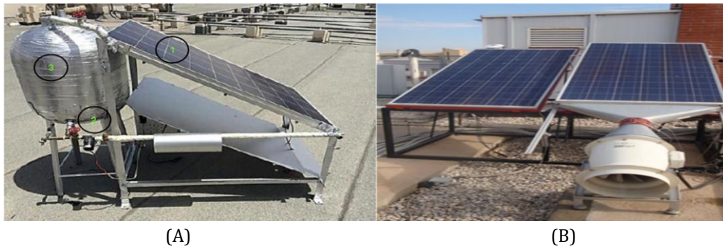
Fig – 7: Hybrid solar Photovoltaic/Thermal (PV/T) systems - (A) cooled by forced water circulation (B) cooled by forced air circulation [ (44), (45)]
