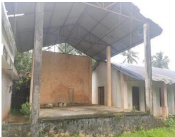
Fig -2 Corroded roof
