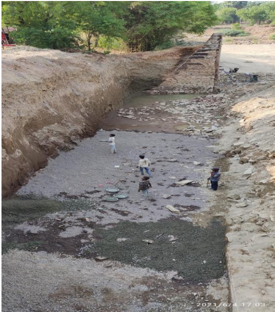
Figure 6 Quarry spall along with lean concreting layer
