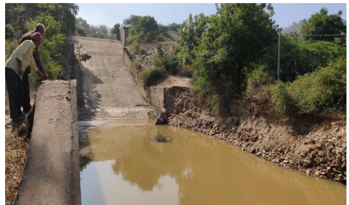
Figure 2 Collapsed part of the Transition wall
