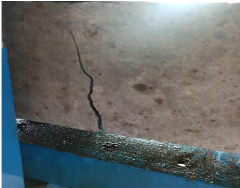
Fig -2: crack pattern on conventional beam
