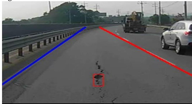
Fig - 4: Pothole Detection
