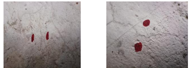
Fig -4d: Fully healing of crack at 28 days
