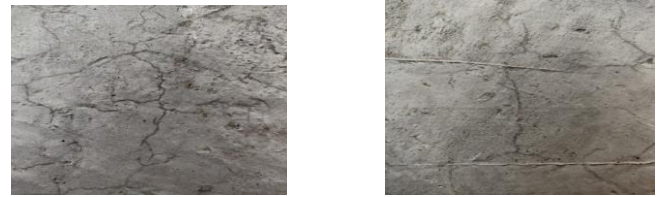
Fig -4b: Partial healing of crack at 7 days
