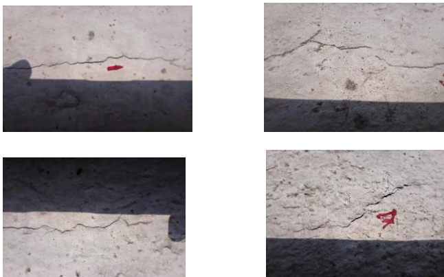
Fig -4a: Initial Crack in Fresh Concrete
