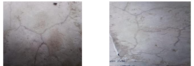
Fig -4c: Partial healing of crack at 14 days
