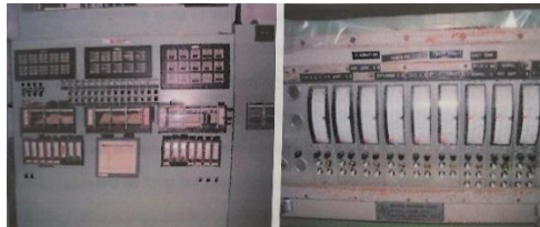
Fig-7: Control panel of Air compressor
