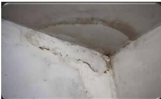
Fig 5 Leakage from corner of slab
