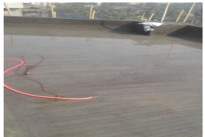
Fig -5: Water ponding after complete of IPS
