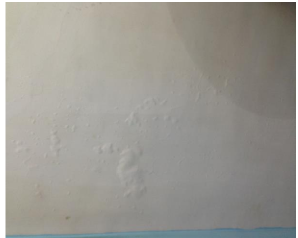
Fig -2: Leakages observed
