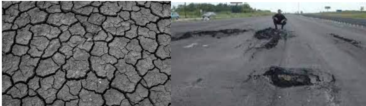
Figure 1: Black Cotton Soil Cracks || Source [3]
