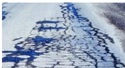
Fig- 3: Freeze thaw deterioration
