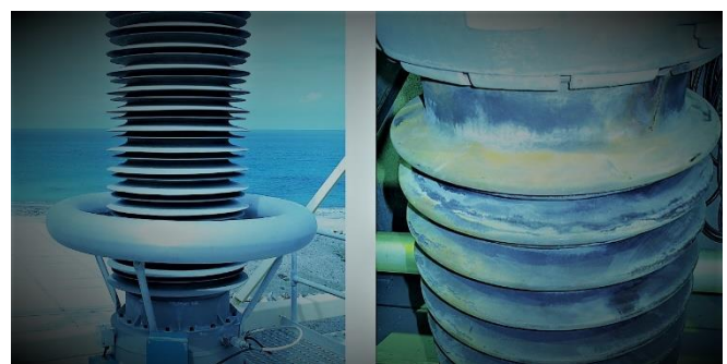
Fig -10: Pollution on insulator
