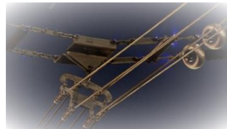
Fig- 9: corona discharge on transmission line
