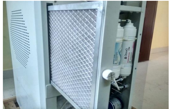
Fig -4: Airfilter installed in ApaH
