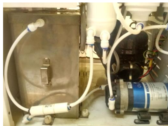
Fig-5 : Lower tank and Booster pump
