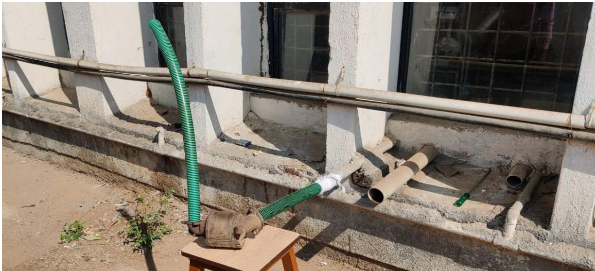
Fig -2: CC connected to exhaust pipe
