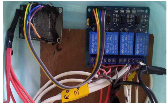
Fig -3: Signal Controller
