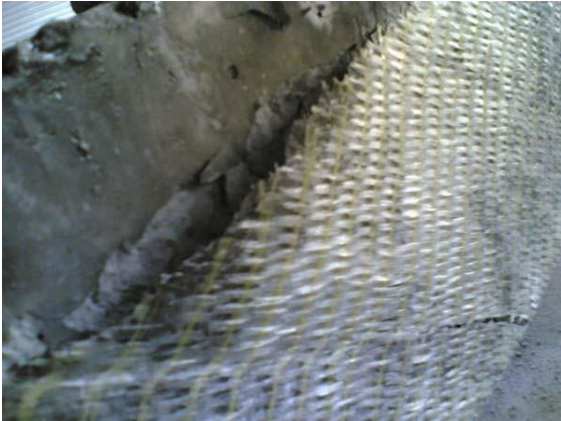
Fig-4 Debonding of GFRP Jacketing with fibers at 45 Degree to the Longitudinal Axis of Beam
