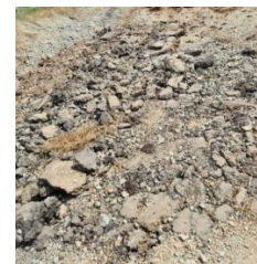
Figure-1: Dumped RAP material
