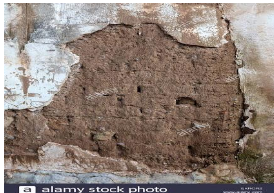
Fig - 2: Old Medieval Plaster
