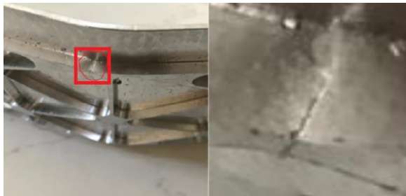
Figure -8: Crack images in the experiments
