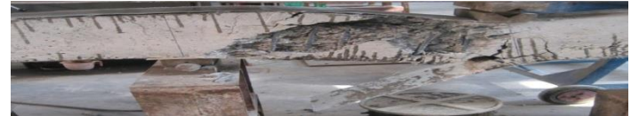
Figure 3.16 Magnified view of the failure of the beam
