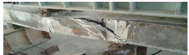
Figure 3.18 Ultimate failure of beam by debonding of FRP with concrete cover
