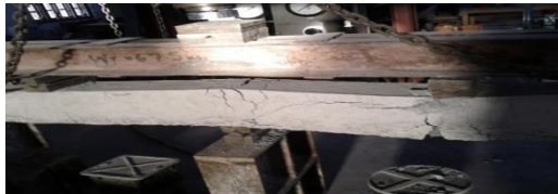
Figure 3.13 Control Beam, CB2 after failure
