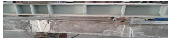
Figure 3.17 Tensile rupture of FRP at mid section of right span at lower value of load
