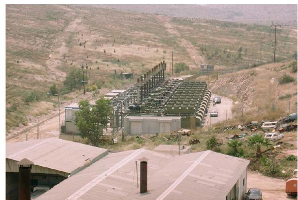
Fig -14: Ano Liosia Landfill gas exploitation project, Athens, Greece
