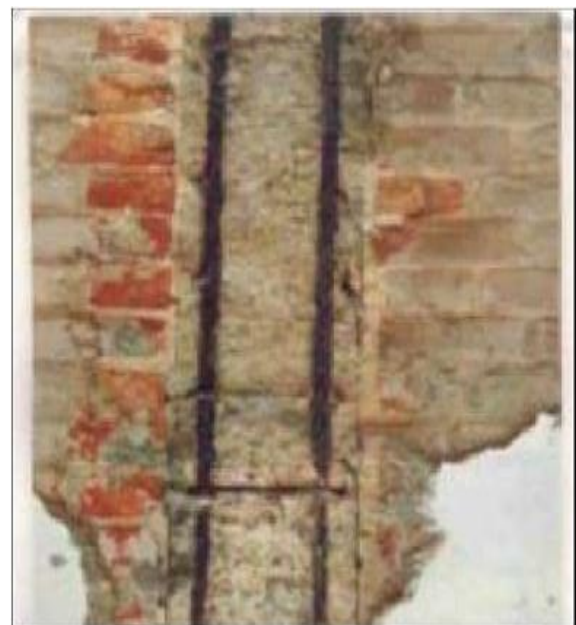
Fig. 02 Spelled cover concrete & exposed cover Reinforcement (Ref. Google)
