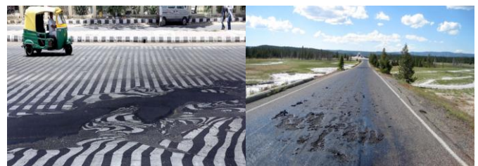
Figure 2.1.2: Deterioration of Bituminous Seal Coat Due to Excessive Heat
