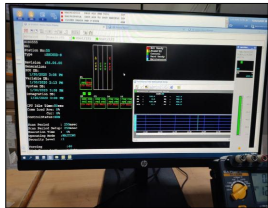
Fig -5: PSU redundancy Check
