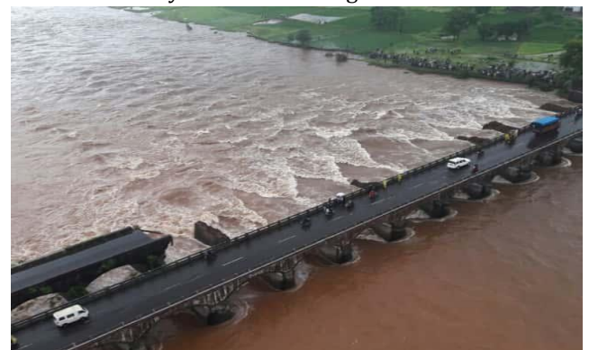
Fig-1: - Bridge Collapse due to flooding at Mahad over Savitri River
