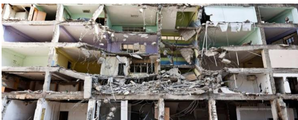
Fig -1 Damages to the building during earthquake
