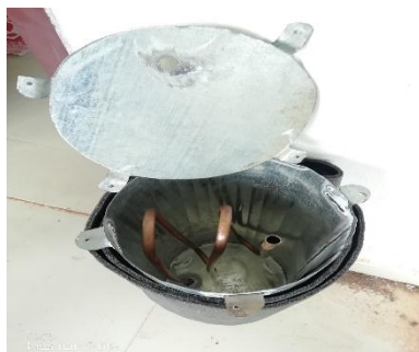
Fig -1: Energy Storage Unit
