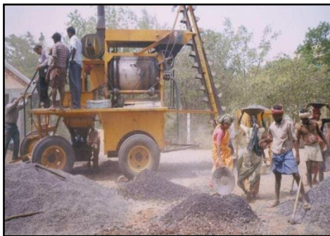
Fig. 2: Heating of Aggregate to 170° C in Mini Hot Mix Plant
